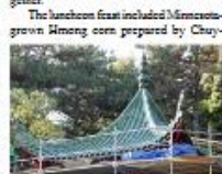
Artisans meet their goal of getting roof completed before they return to China.
